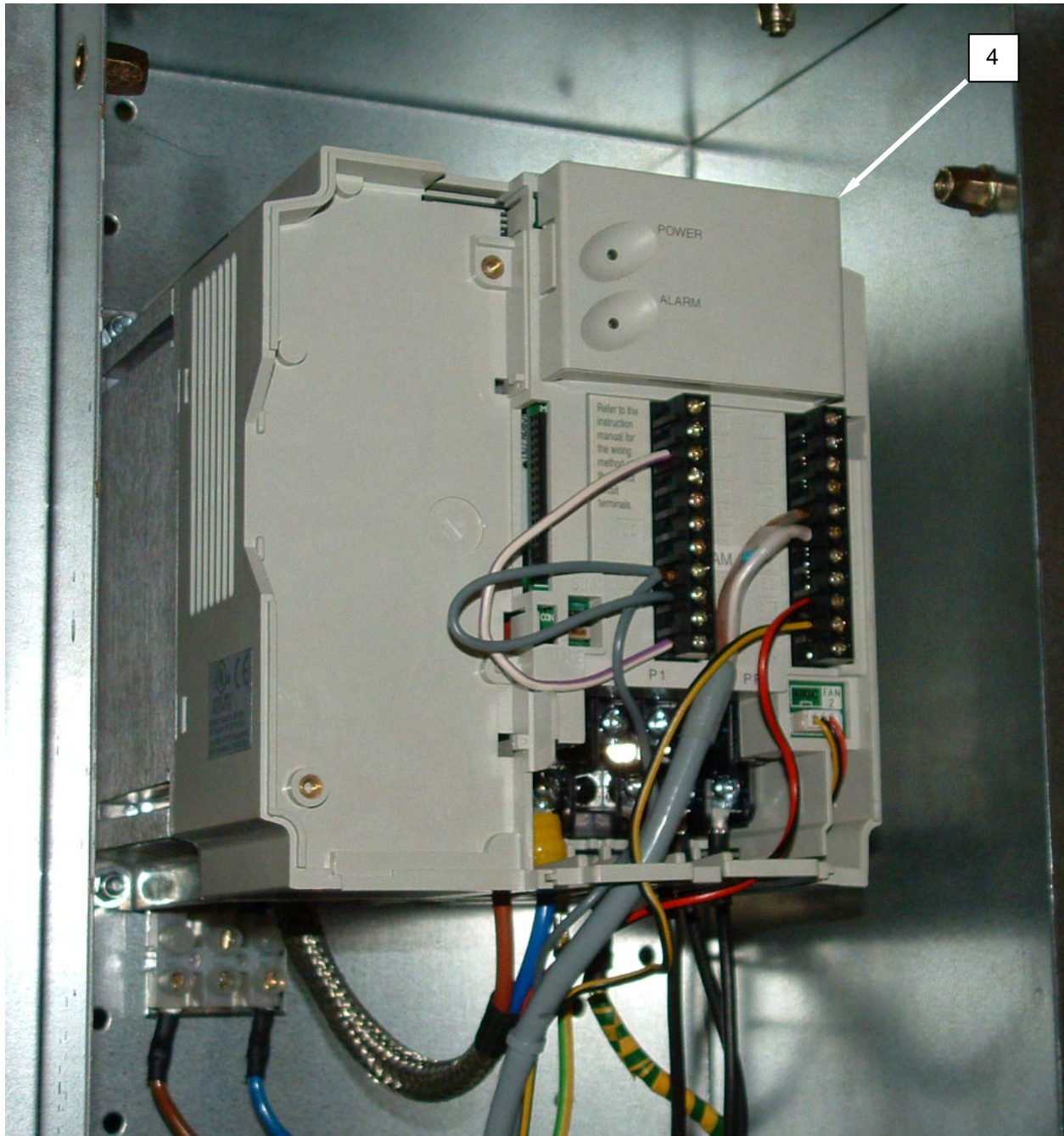
Figure 2. Replace the Washer Variable Frequency Drive (Sheet 2 of 2).
