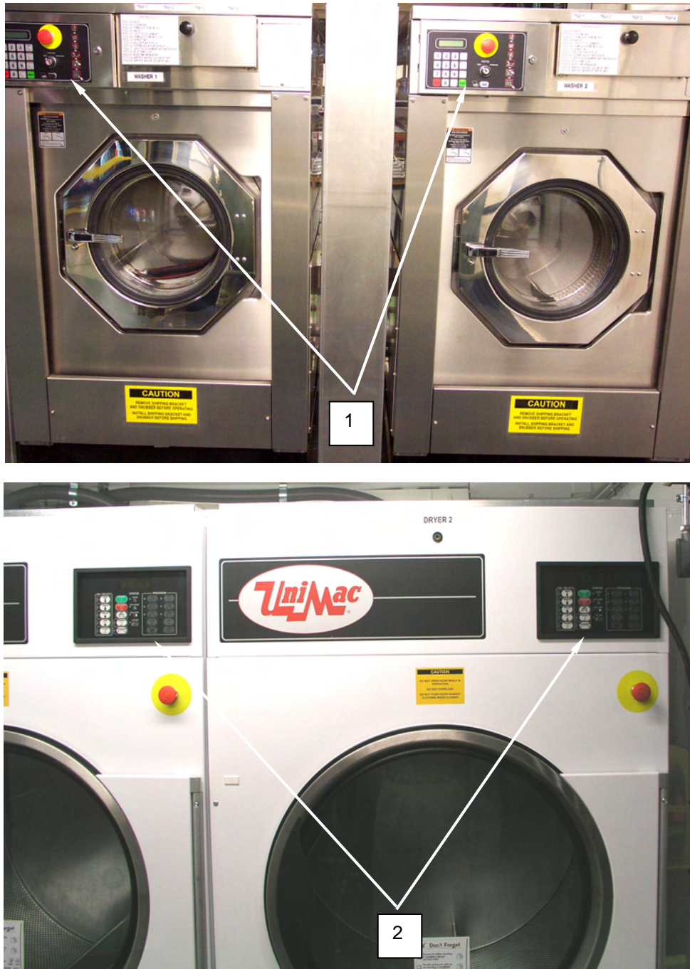
Figure 10. Washer and Dryer Control Panels.
