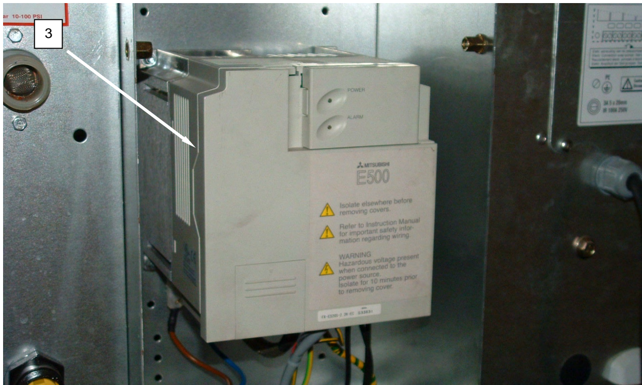
Figure 2. Replace the Washer Variable Frequency Drive (Sheet 1 of 2).
