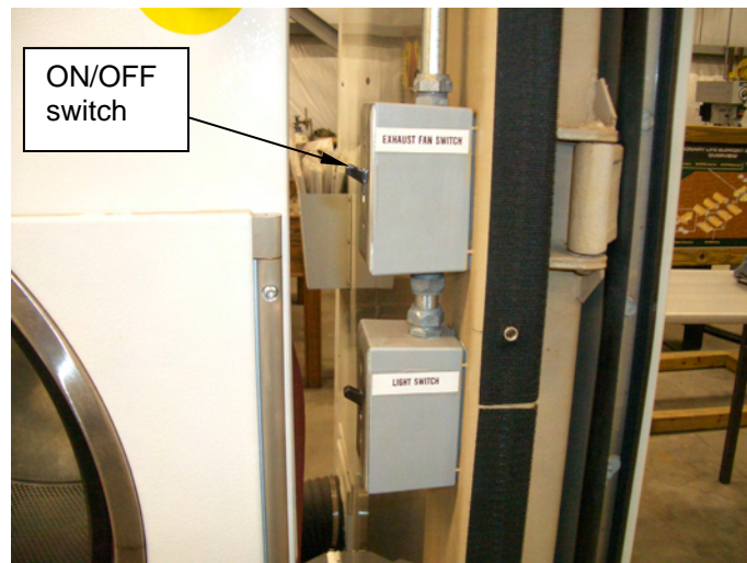
Figure 31. Shutting Down Exhaust Fan.
