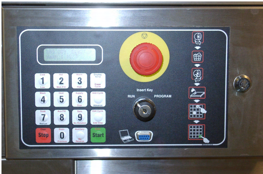
Figure 1. Test the Variable Frequency Drive.
