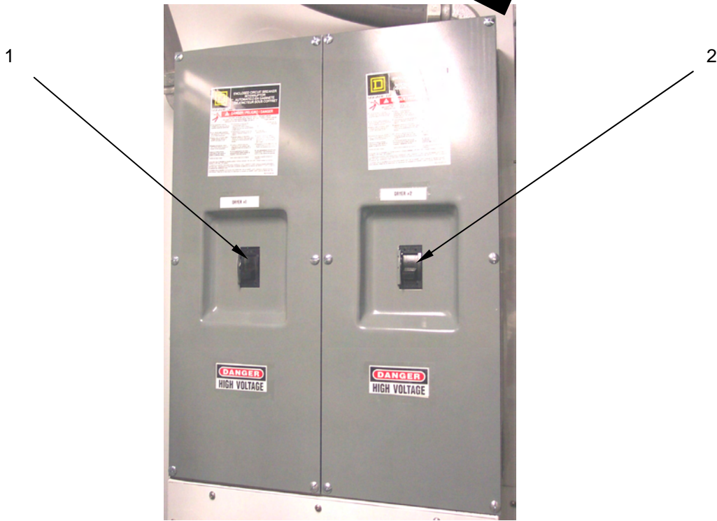
Figure 6. Dryer Circuit Breaker Panel.
