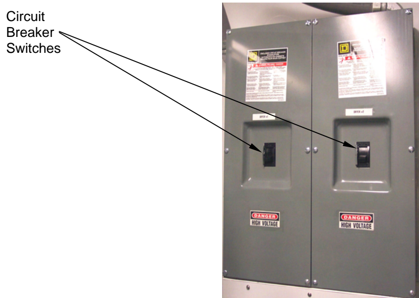
Figure 18. Set Breakers to OFF.
