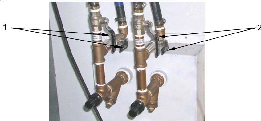
Figure 1. Hot and Cold Water Shutoff Valves.
